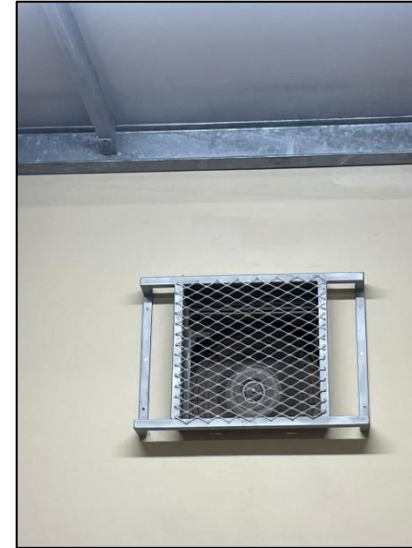
6. Chemical store fitted with appropriate extraction
