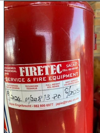
8. Fire extinguishers recently serviced and available where needed
