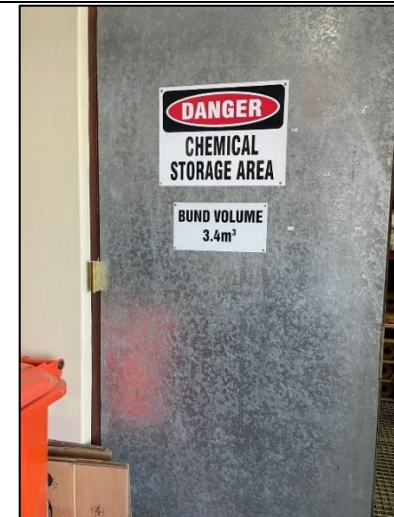
4. Purpose built banded chemical store
